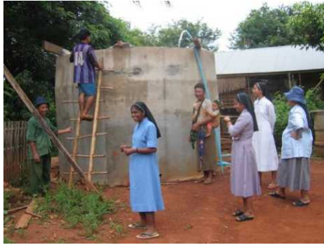
Water Tank in Hway Thar 2 Village
