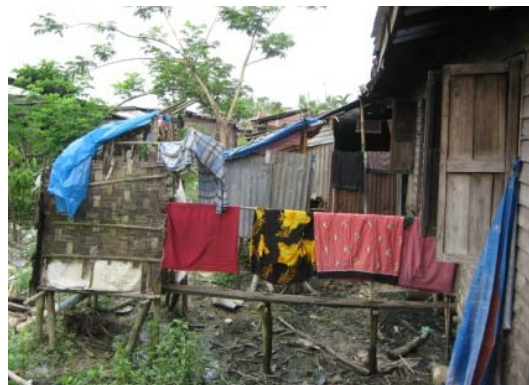
Dilapidated Nursery Building (Dala)
