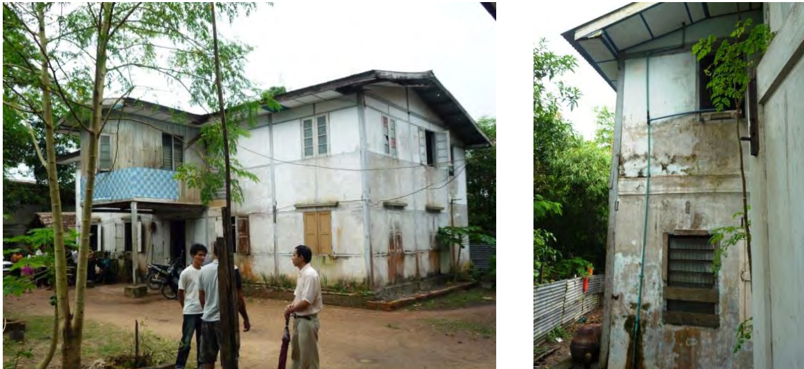
The crumbling and mouldy house of St. Bruno Orphanage
